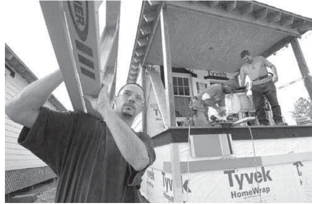
A work crew constructs a house that the Southern Mutual Help Association helped finance. Photo courtesy of SMHA.
